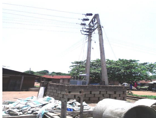
The transformer donated to Okin village (Authors' field work, 2014)
